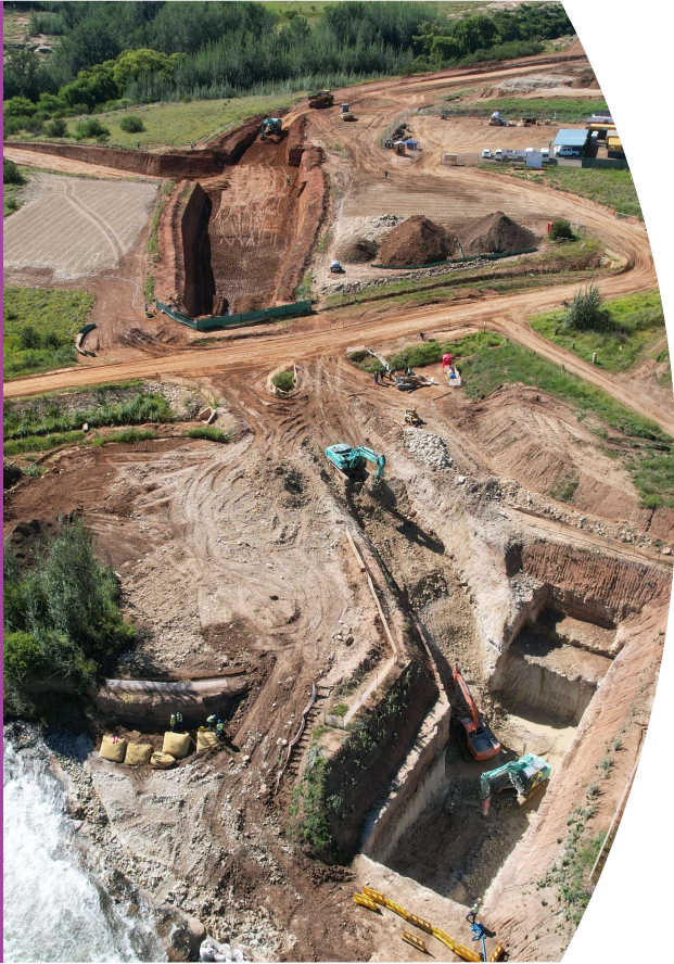
Hydro Plant in Clarens
